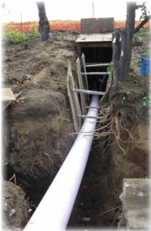
The recycled water distribution project featured a number of unique and challenging design elements, including sliplining over 6,900 feet of an abandoned raw water line with fusible PVC pipe.
