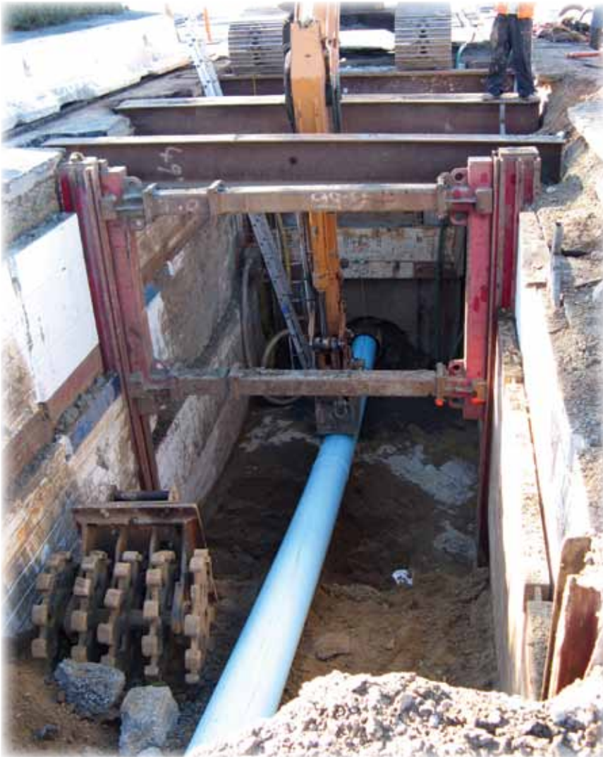
Jack and bore construction was used to cross beneath W. Antioch Creek on W. 10th Street. The top of the pipe is about 16 feet below grade.
