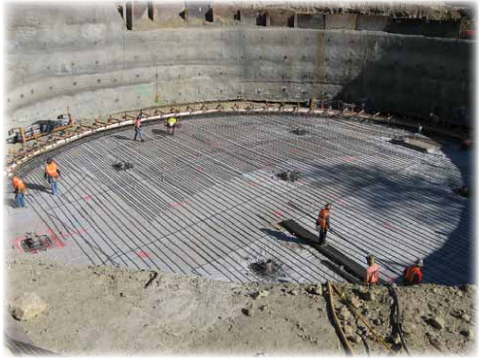
The project includes construction of a 1.1 million gallon reservoir and pump station at the golf course.
